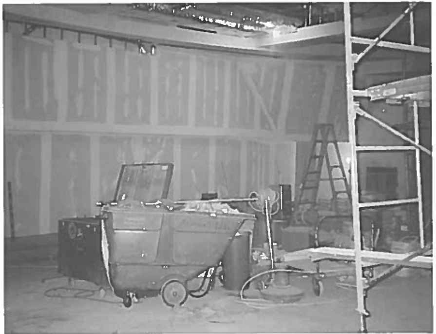
Do you recognize this space? You should—it's the main lecture hall, room 228, getting a complete renovation.
