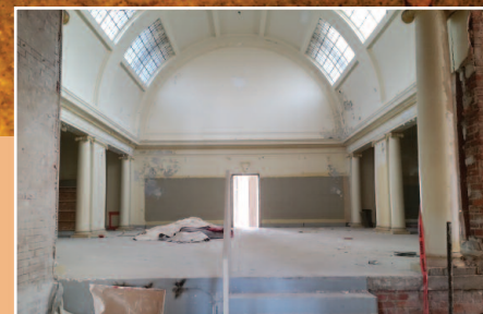
Interior of the previous museum space, which will be the new student hub when NHB reopens.
